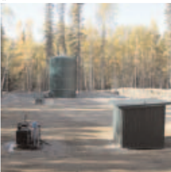
Evergreen's Stromberg production facility in the Mat-Su Valley includes a 400-barrel production tank and meter shed. The facility has containment berms with impermeable liners. (Photo by Judy Patrick)
