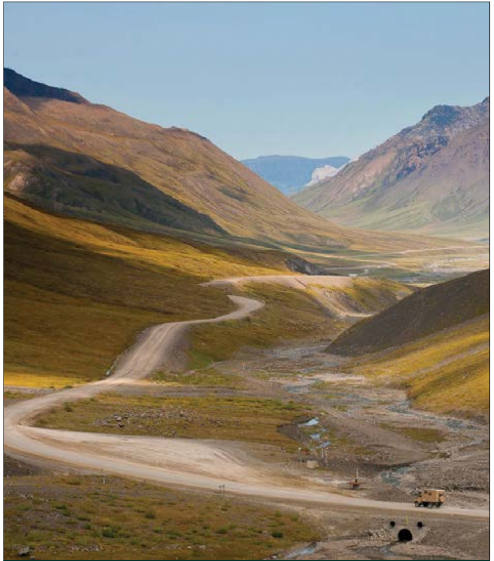
Dalton Highway in the Brooks Range. Permafrost thaw is creating problems for the roadbed.
