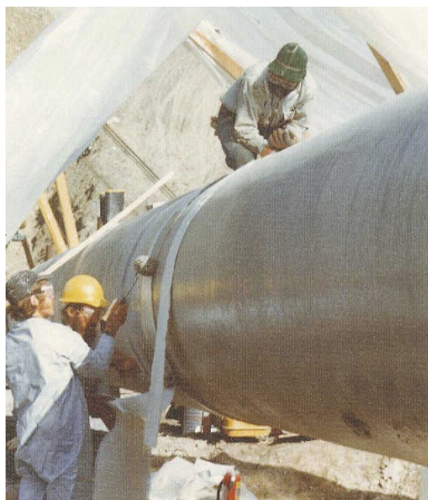
Crew insulates a joint on the pipeline north of the Yukon River in the summer of 1976.
