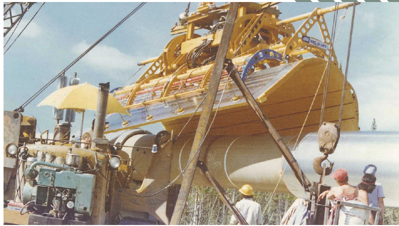
TAPS construction near the southern foothills of the Brooks Range in 1976. Oil from the North Slope and the pipeline that carried it brought great wealth to Alaska. (Photos by Carl Portman)
