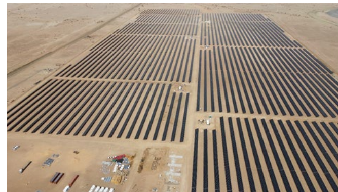
Tasiast – Solar PV plant with 34 MW capacity
